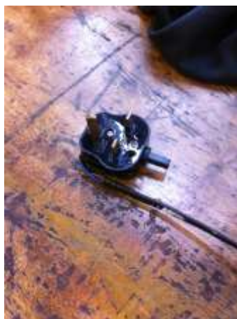
Sat 12 th Oct, power cable/socket broken
